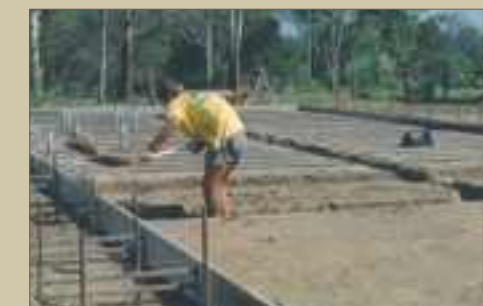
With the Camilleri System installed prior to construction, this dwelling (left) will be protected from termite attack for the rest of its life without having to drill the slab for future treatment.
