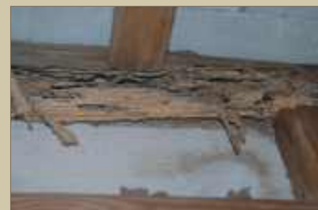
This Termite infestation is typical of homes constructed on a concrete slab, many within the first 12 months following construction.
