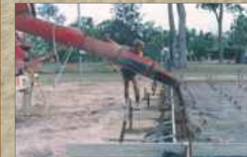
At left: Moisture is retained under the polythene membrane which in turn is a major attractant to Subterranean Termites
